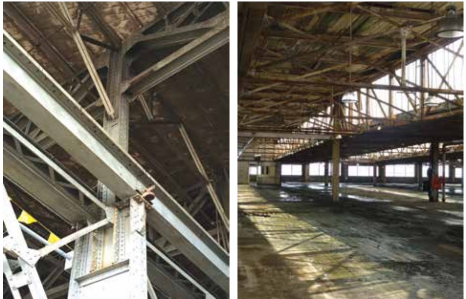
Figure 3. Complex existing conditions at the first story (left) and roof trusses (right).
