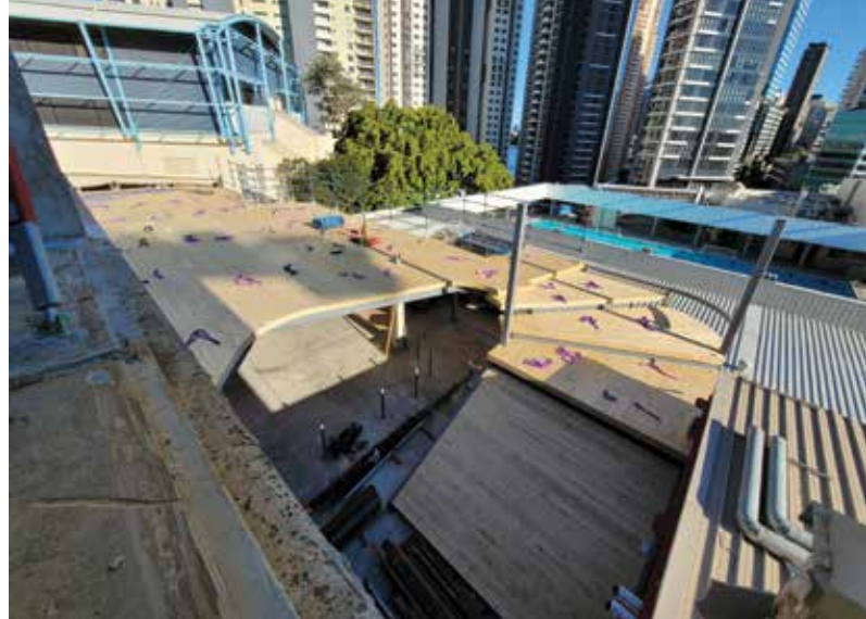
The reading stair. Level 03 under construction with a large void and feature reading stair.
