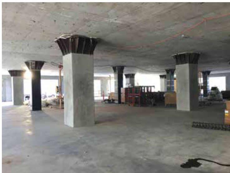
Figure 3. Column Retrofits – Existing interior columns are strengthened with a shotcrete jacket or CFRP wrap. All columns are topped with steel collars to catch the slab in the event of a punching shear failure.
