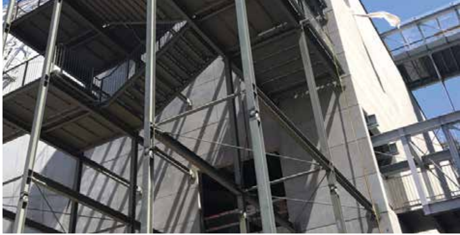
In an earthquake, the theater building moves on the base isolators below, and these hinges allow the stair columns to "lean over" so that the upper portion of the stairs can go "along for the ride." These joints are hinged in two perpendicular axes, effectively allowing rotation and translation in any direction.
