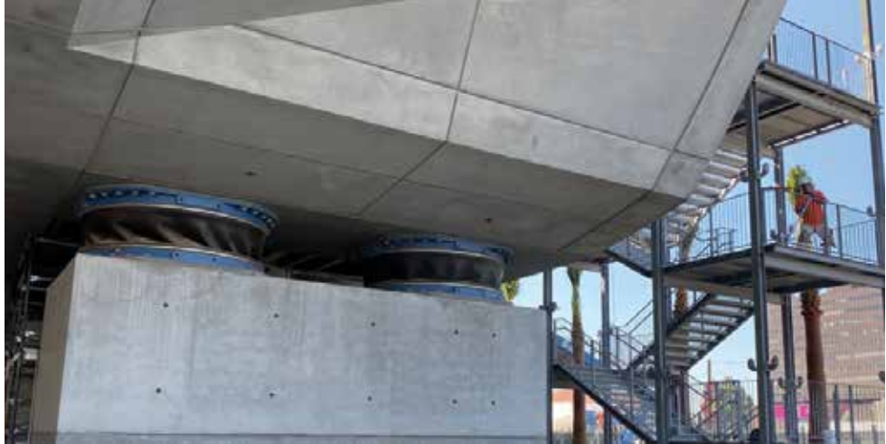
In an earthquake, the spherical theater building moves on a novel base-isolation system with four mega-columns in a system that seismically isolates the structure from the ground.
