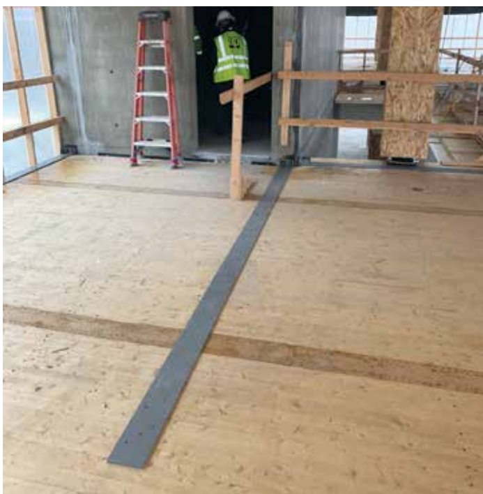
Figure 7. Collector strap from CLT diaphragm to core walls at Platte Fifteen building in Denver, CO (Oz Architecture/KI&A Engineers and Builders). Courtesy of JC Buck.
