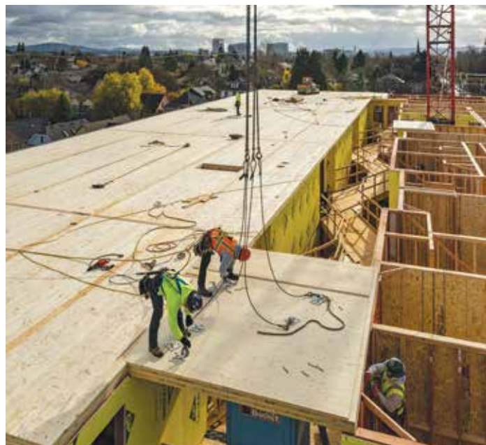
Figure 2. Panel-to-panel connections with splines at The Canyons building in Portland, OR (Kaiser+Path). Courtesy of Marcus Kauffman.
