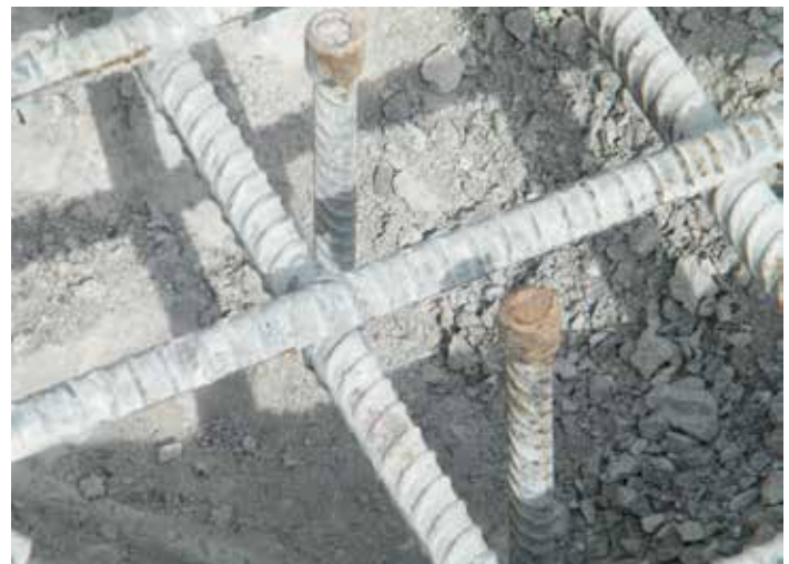
Figure 9. Reinforcing bar coupler that failed in direct tension.
