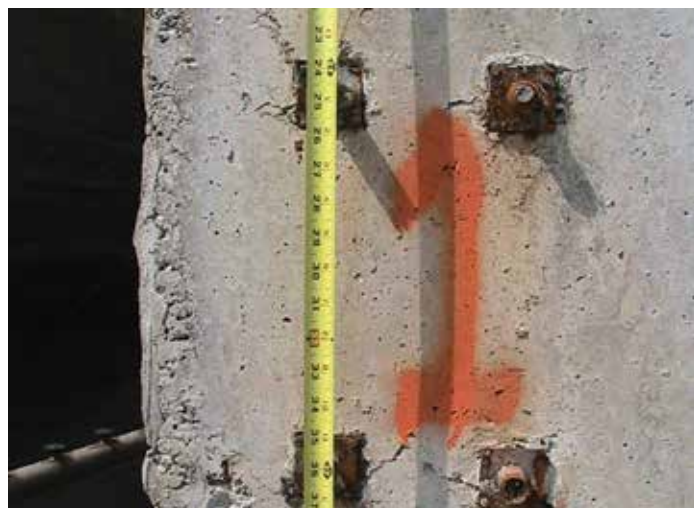
Figure 8. Reinforcing bar couplers and location where reinforcing failed in direct tension.
