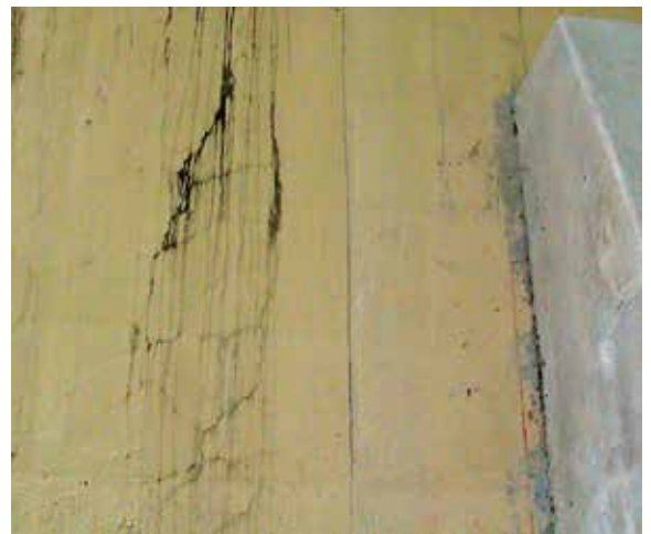
Figure 3. Cracks in the north wall caused by the excessive displacement of the wall. The added buttress is shown to the right of the photo.
