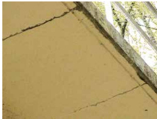
Figure 4. Cracks in the upper walkway along the north wall. This was caused by the excessive displacement of the wall.
