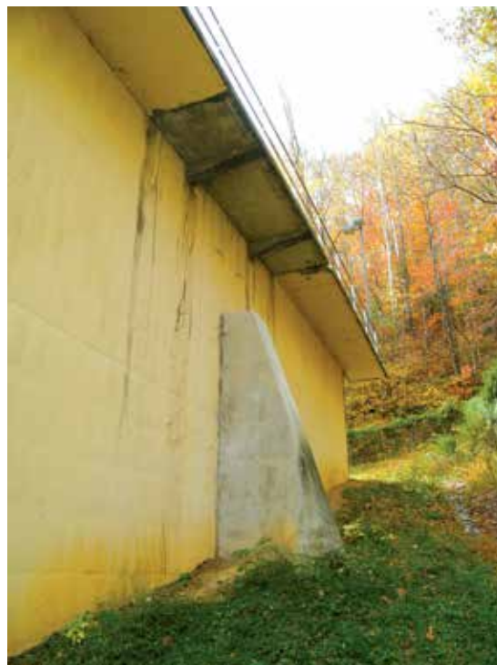
Figure 5. Concrete buttress that was installed along the north wall of the basin shortly after the basin was placed into service. The wall is cracked in the area in front of the buttress.
