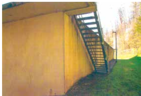
Figure 6. View shows the structure's west wall and evidence of overflow and wastewater to a height of 30 feet 5 inches in the basin.
