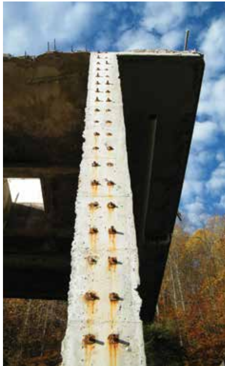
Figure 7. Looking up at reinforcing bar couplers placed at the east end of a baffle wall. The couplers are placed at 12-inch vertical and 7-inch horizontal centers.
