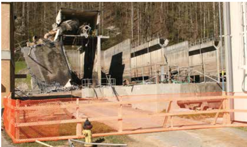
Figure 2. Front view showing the collapsed east wall of the Gatlinburg Wastewater Plant equalization basin.
