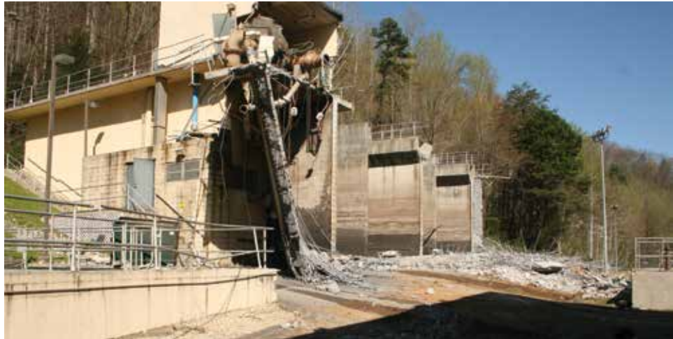
Figure 1. Overall view of the collapsed east wall of the Gatlinburg Wastewater Plant equalization basin looking from south to north.
