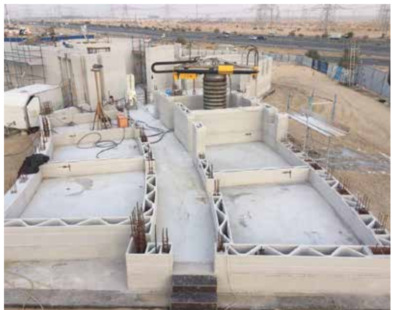
Figure 4. Under construction, a modern 3-D printed building features relatively conventional reinforcing and a radial printing system built by Apis Core. Courtesy of Apis Core.
