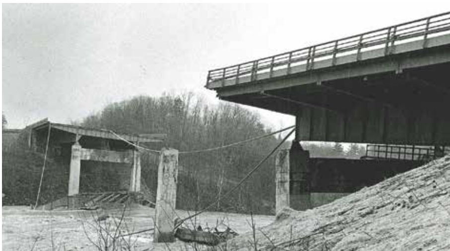
Bridge with three spans out.
