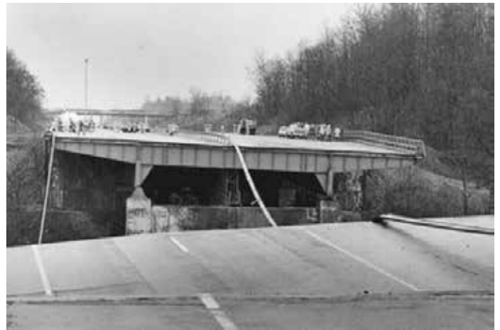
The Schoharie Creek Bridge collapse.
