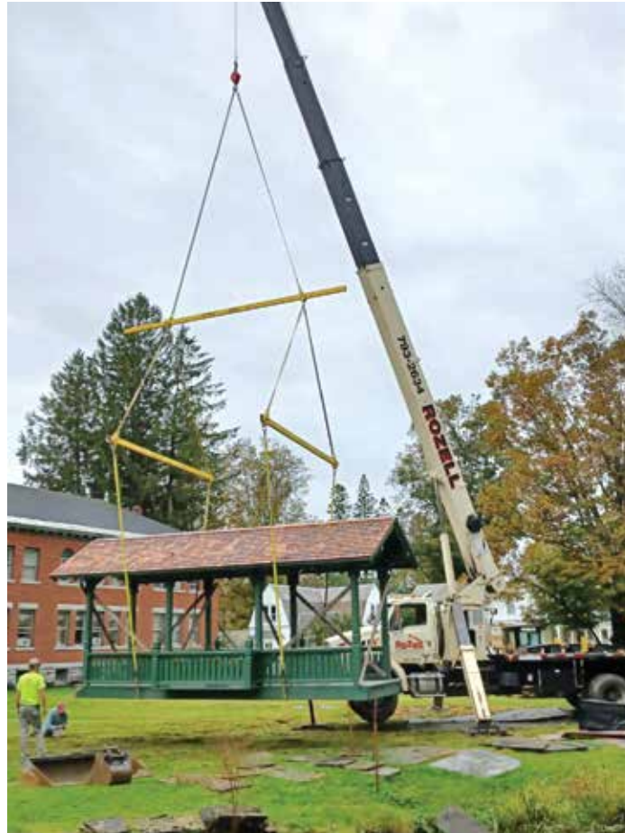
Bridge being set on new abutments with the help of donated crane services.
