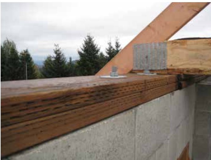
Anchor bolts are used to attach the top plate to the masonry wall.
