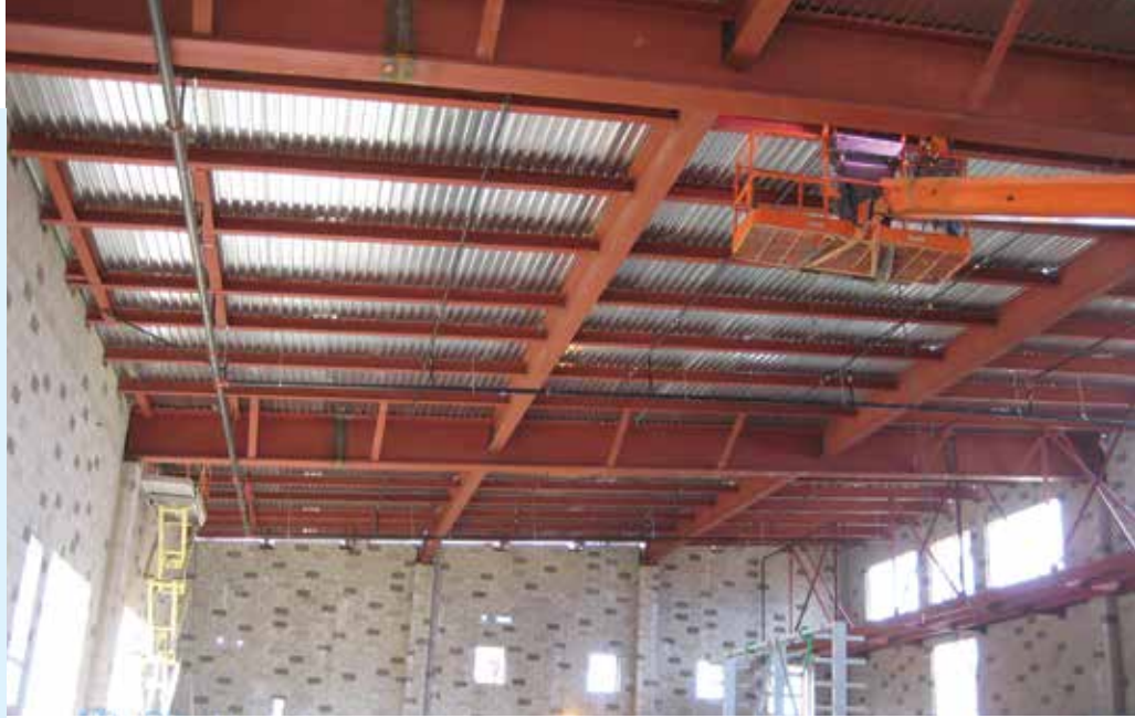
Numerous anchor bolts are required in this structure to attach the roof to the masonry walls.
