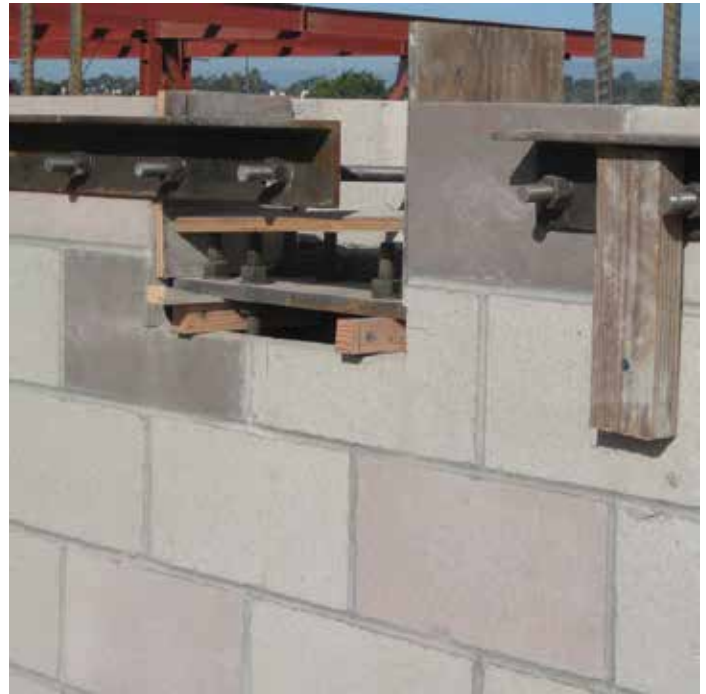
Anchor bolts are used to attach the ledger angle to the side of the masonry wall. Additional anchor bolts are used in the beam pocket for the base plate. Note that the ledger angle was installed over the face of the beam pocket, which had to be amended in the field.
