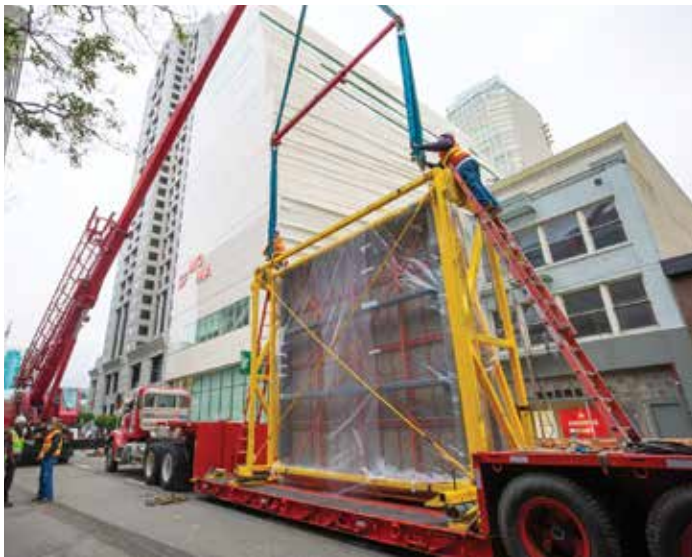
Figure 3. Existing panel frame (orange), panel mount (gray), travel frame and cart (yellow), and wire rope isolators (gray) on the truck bed.
