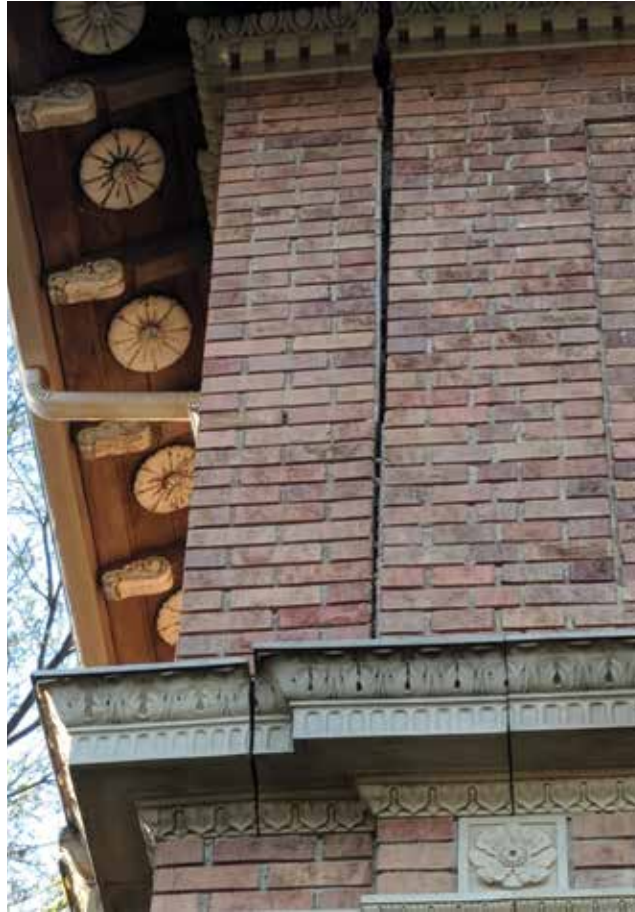
Figure 3. Cracking at the southwest corner.
