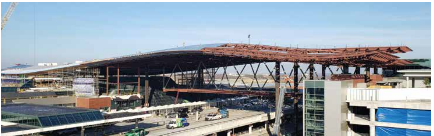
The new terminal roof was lifted a few feet to span over the existing occupied terminal and roadway – offering tremendous structural, architectural, and construction benefits.
