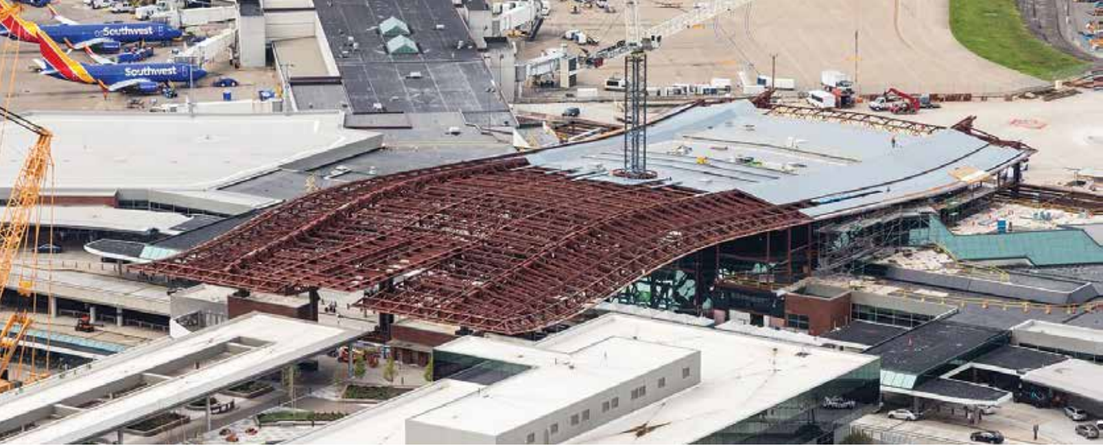
At Nashville International Airport, the new roof's unique, mildly rippled form is created with just two curvilinear spine trusses. Courtesy of Aerial Innovations Southeast.
