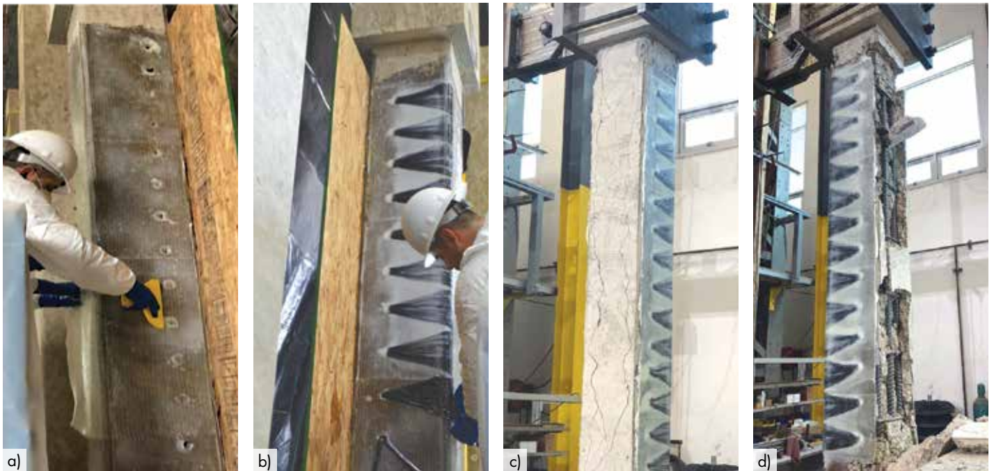
Figure 15. a) Installation of three-sided FRP wrap, including drilled holes that receive the FRP through-anchors. The holes are countersunk in a trumpet shape at the column; b) Installation of the FRP through-anchors, showing the splaying of the carbon fibers of the anchors onto the first layer of FRP wrap; c) Retrofitted column tested parallel to through-anchors, shown after reaching a peak lateral story drift ratio of 5.5% to the left followed by 11% to the right; d) Retrofitted column tested perpendicular to through-anchors, shown after reaching a peak lateral story drift ratio of 5.5% to the left followed by 11% to the right.
