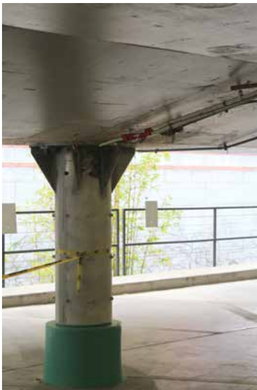
Figure 4. Steel jacking of the existing concrete column at the parking structure level.
