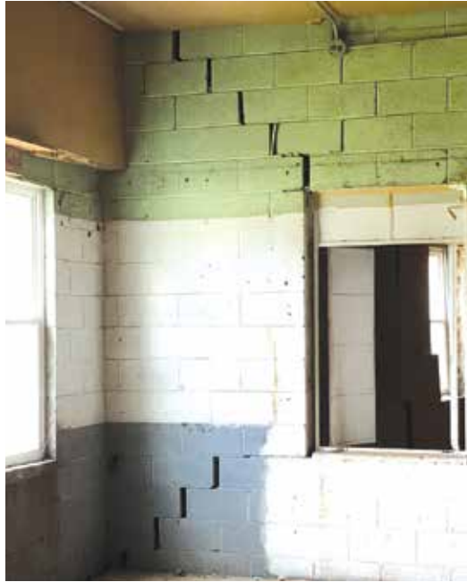
Displacement of unreinforced masonry at an industrial building in Sparta, NC, following the August 9, 2020, earthquake.
