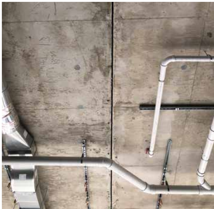
Figure 4. Standard PS=Ø application where the second slab is poured directly against the first slab; all MEP and curtain wall trades have worked without delay across the bottom of this SRJ at the Even Hotel in Rochester, MN.
