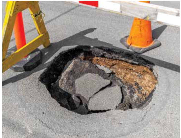
Figure 1. Sinkhole caused by TBM tunneling work.
