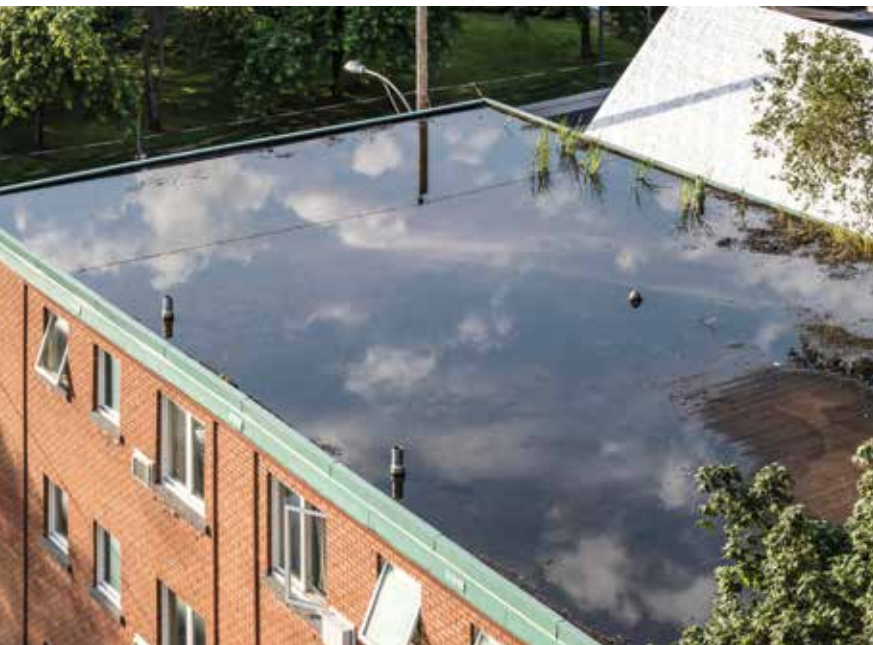
Figure 2. Design for ponding instability is based on secondary drainage system rain loads.
