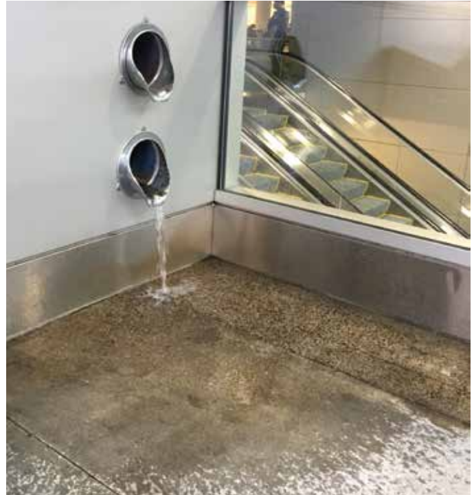
Figure 1. Secondary drainage system outflow.
