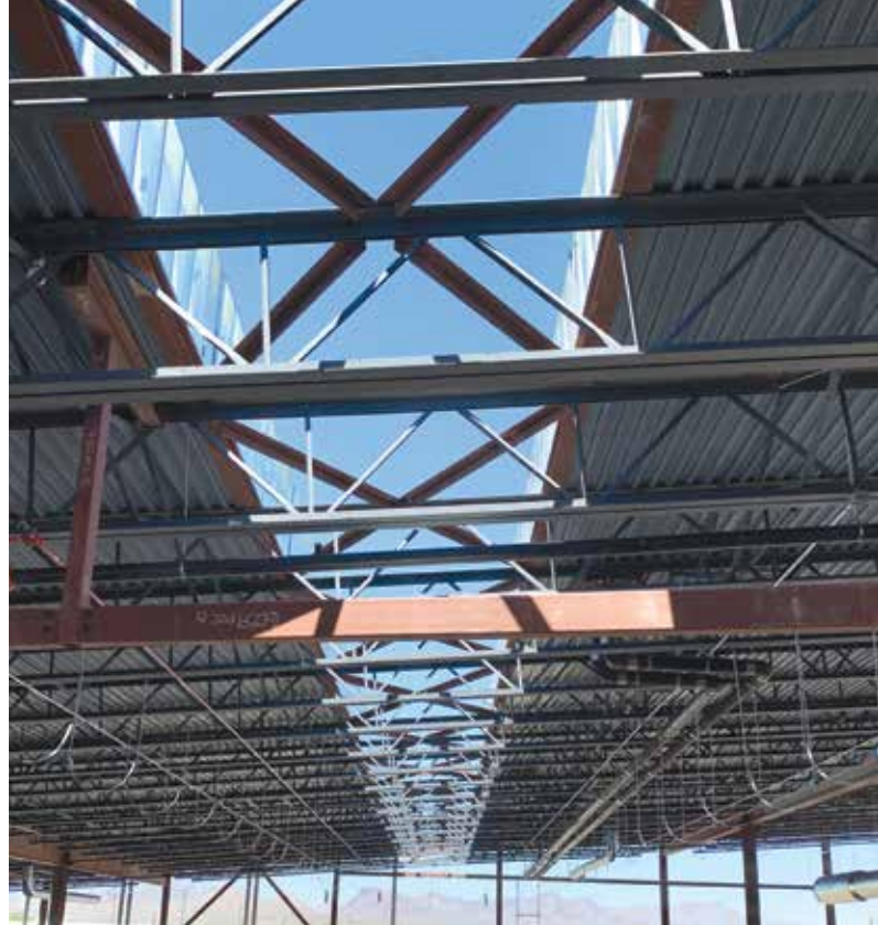
8. 5-foot-wide skylight illuminates the high-volume work bay.
