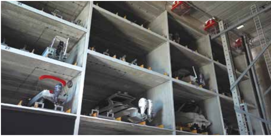
In an automated dry boat storage facility, the structural design must consider the additional weight of fire suppression water, which may collect in the stored boats in the event of a fire.
