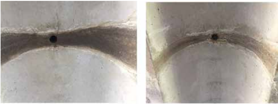
Figure 4. Water damage at mid-span.
