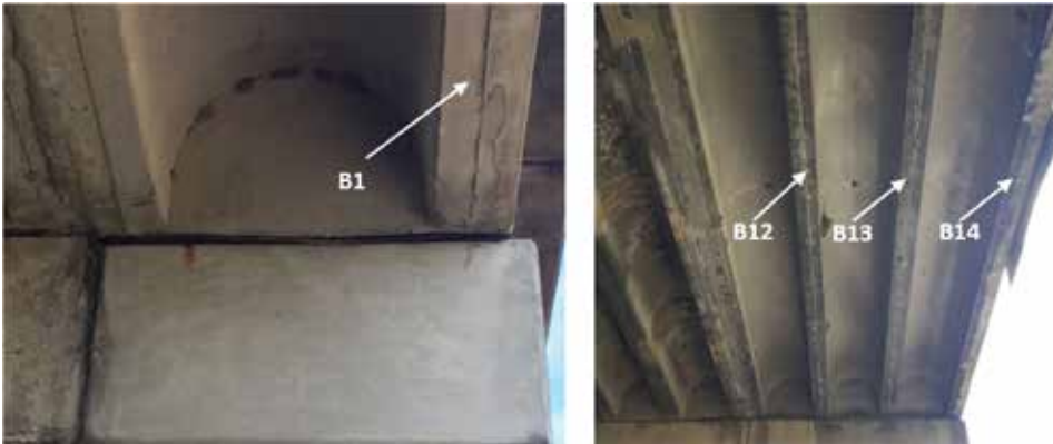
Figure 5. Condition in newer beams.
