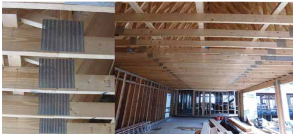
Metal plate connected wood trusses and punched sheet metal plate connectors.
