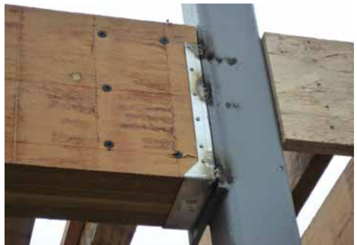
Wood-to-steel column connection. Weld material reaction to paint.
