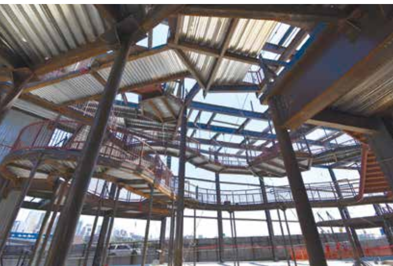
Figure 3. The interweaving catwalks and viewing platforms caused the structural design team to consider the effects of differential and compound deflections along these catwalks.
