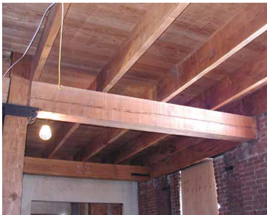
Figure 2. Timber beam with checks in a 100-year old construction. The checks were limited in size once the timber acclimated to in-service conditions.
