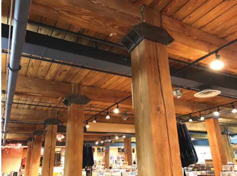
Figure 6. Seasoning checks that reveal the natural characteristics of large timbers are often desired for a rustic appearance.
