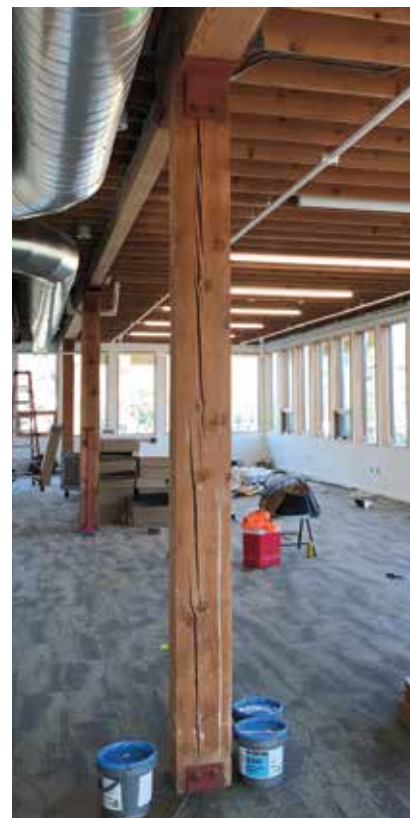
Figure 1. Timber column with seasoning checks in construction. The timber acclimated to in-service conditions.
