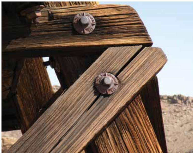
Figure 5. Seasoning check that developed into a split due to a bolted connection where tension perpendicular to grain stresses results from the bolt acting as a wedge.
