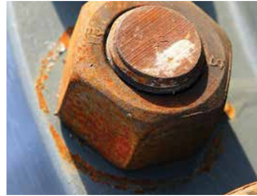
Figure 1. Corrosion of connections is a common concern.
