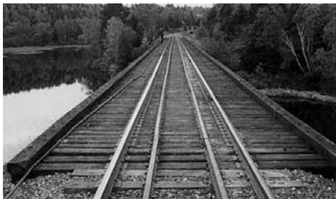
Wooden trestle with the recommended steel guardrails, closely spaced ties, and wooden outer rails.
