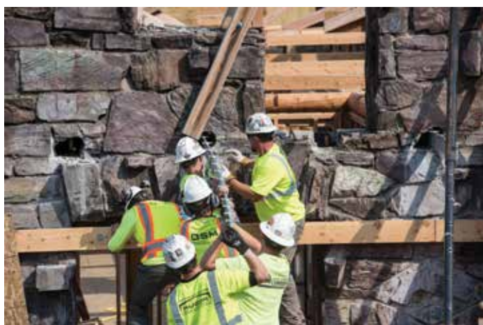
Figure 8. Construction crew fishes second-floor balcony's joist fitch through wall pocket. Courtesy of A Boring Photo.
