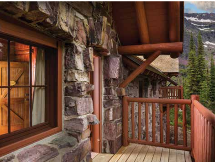
Figure 6. Completed roof and balcony framing as well as rehabilitated masonry. Note unremovable soot stain over door. Courtesy of Mark Bryant Photographics.
