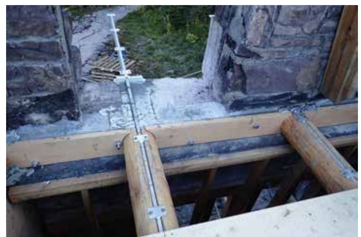
Figure 9. Second-floor balcony joist fitch grouted in wall pocket. Joists are supported on inside face of wall by a steel angle ledger.
