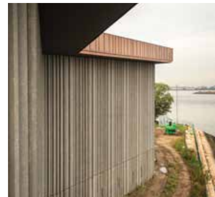
The museum's exterior's vertical ribbed pattern took some cues from the nearby Palisades cliffs in New Jersey that have a vertical rhythm. Credit: Frank Linemann, courtesy of FXCollaborative.
