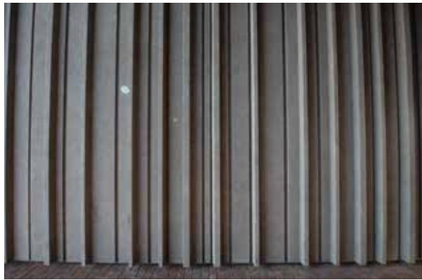
A form-liner imparted a deep vertical relief creating shadow that the design team wanted, its darkness to accentuate the panels and complement the context and site. Courtesy of Timothy Schenck Photography.
