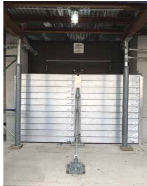
Figure 1. Training exercise: Deployment of an aluminum flood plank system. Courtesy of Angelica Chan, STV.
