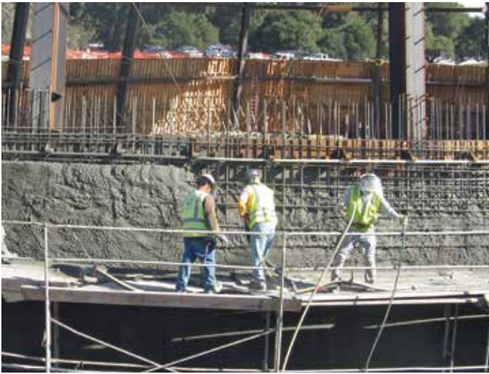
Shotcrete placement on the Bing Concert Hall. All concrete placement fully visible during shooting. Courtesy of Joseph J. Albanese, Inc.
