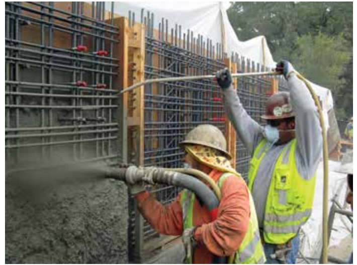
ACI-certified wet-mix shotcrete nozzleman shooting a structural mockup panel. Courtesy of Joseph J. Albanese, Inc.
