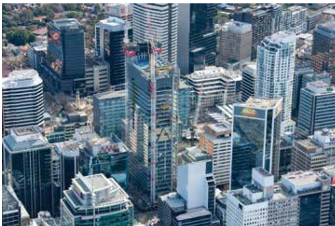
Figure 2. Aerial construction shot of leading western core and following mega-brace. Courtesy of Ethan Rohloff.
