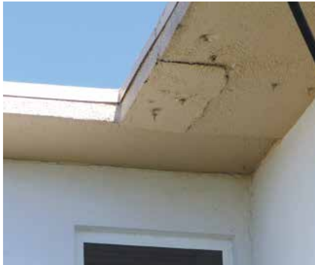
Falling object hazard due to a failed roof membrane over a concrete slab.
