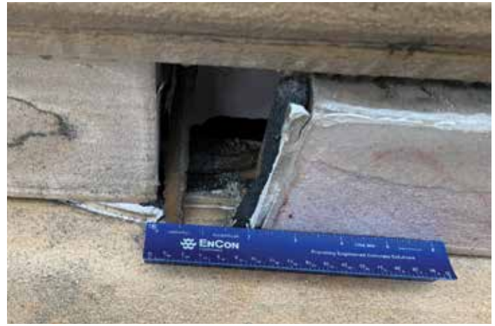
Figure 5. Salt Lake City & County Building – displaced stone at isolated plane.
