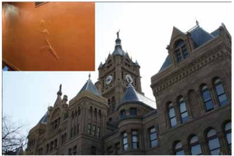
Figure 2. Masonry cracking manifested in plaster coating (inset).
