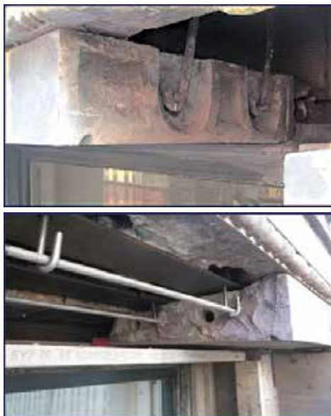
Figure 2. Hung lintel elements. Original construction circa the 1890s (top); repair detail circa 2015 (bottom).
