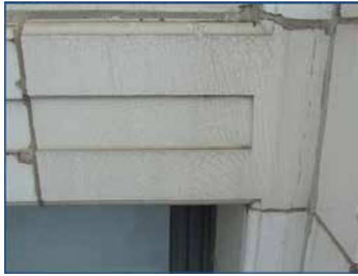
Figure 3. Units with combined support at the pier. Note diagonal stress relief cracks and crazing.
