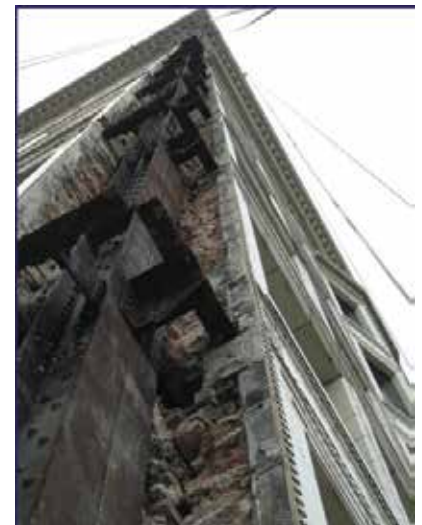
Figure 1. Lack of continuous intermediate support at a corner.
