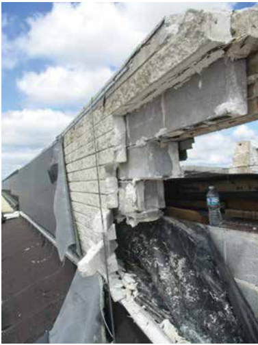
Figure 5. Parapet failure due to lack of anchors at the slip plane of flashing.
