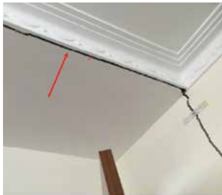
Figure 1. Example of damage due to deep excavation.
