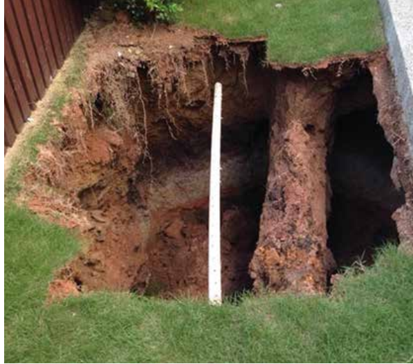
Figure 3. Sinkhole due to ground loss.
