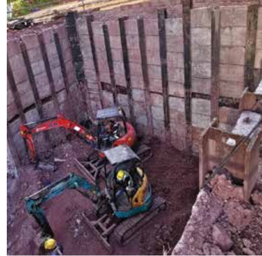
Figure 4. Gaps in soldier piles.
