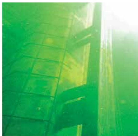
Figure 7. Aligned and welded T 120 structural profiles. Approximately 14 feet of linear weld was placed for the installation of each structural profile T 120.
