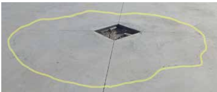
Figure 2. Circular crack around the column block out (highlight added).
