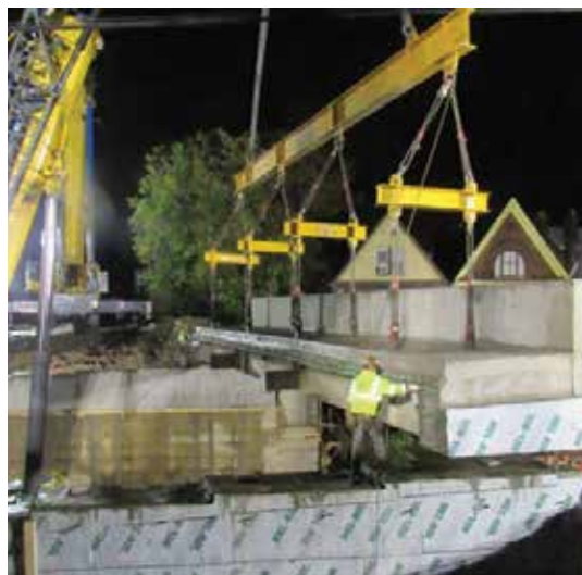
Figure 4. Accelerated Construction of U.S. Route. 30 over Bessemer Avenue in East Pittsburgh, PA. Courtesy of HNTB Corporation.
