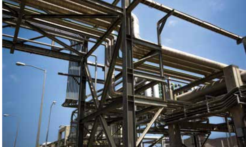
Pipe rack at an oil and gas facility with multiple additions after initial design and construction.
