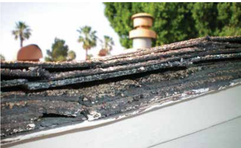
Roofing layers stacked on top of each other, causing structural members to sag under the weight. (photo source: https://bit.ly/3aLYxlc )
