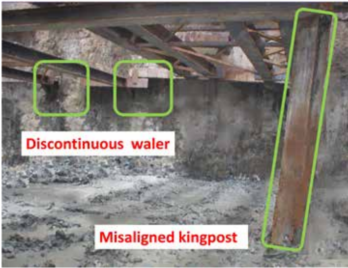
Poor strutting design and construction.
