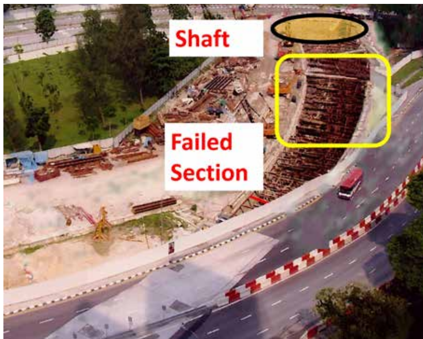
Lateral soil pressure acting on D-wall panels causing joint to open up.
