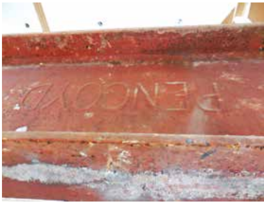
Figure 3. Existing beam from a 1920s building with a "Pencoyd" stamp from the Pencoyd Iron Works.
