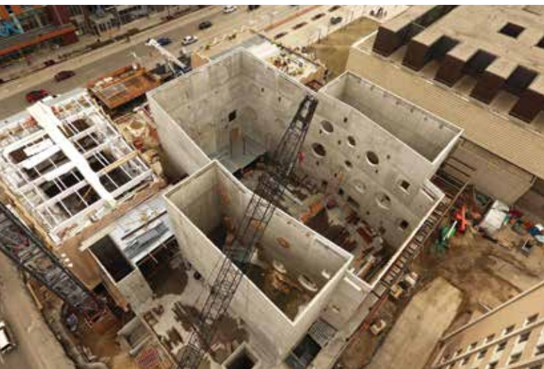
Figure 2. The scale of the reverberation chambers on each side of the concert hall is evident during construction, as are the extensive acoustical openings to the chambers and coffers in the walls overall.
