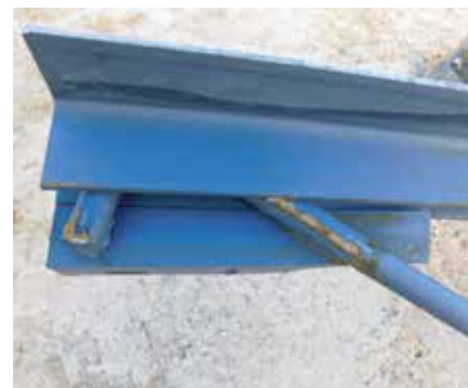
Figure 7. Close-up view of joist seat, which has sheared off at suspect quality weld locations.
