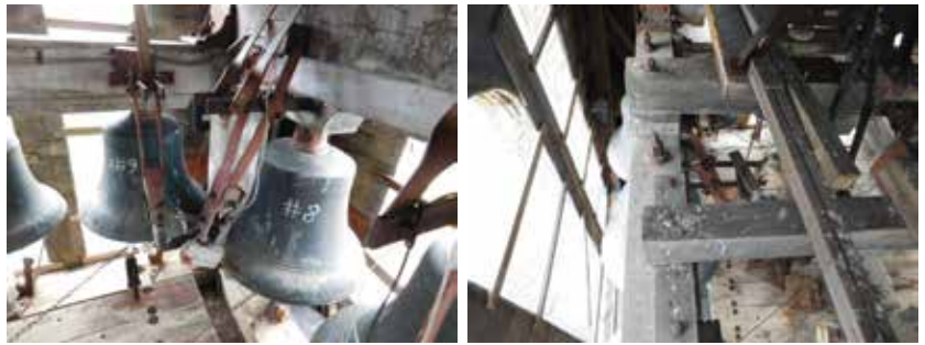
Figure 2. Left: View from the belfry where bells are observed to be permanently affixed and stationary. Right: View from the belfry revealing the bell support framing is structurally isolated from the tower
