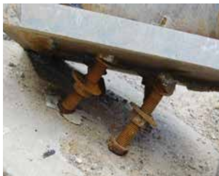
Figure 6. Close-up view of anchor bolt washers and nuts that pulled through oversized baseplate holes.
