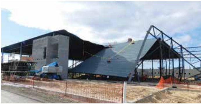
Figure 5. Partial view of framing and roof collapse.
