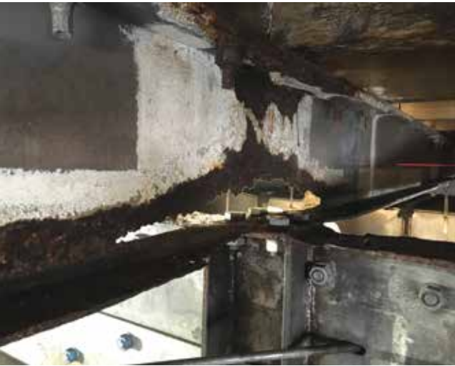
Figure 1. Corrosion of steel beams below the cooling tower.
