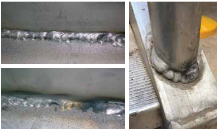
Figure 2. AWS Code D1.2 structural aluminum welds. Welds were rejected due to unacceptable profiles, overlap, and poor workmanship.
