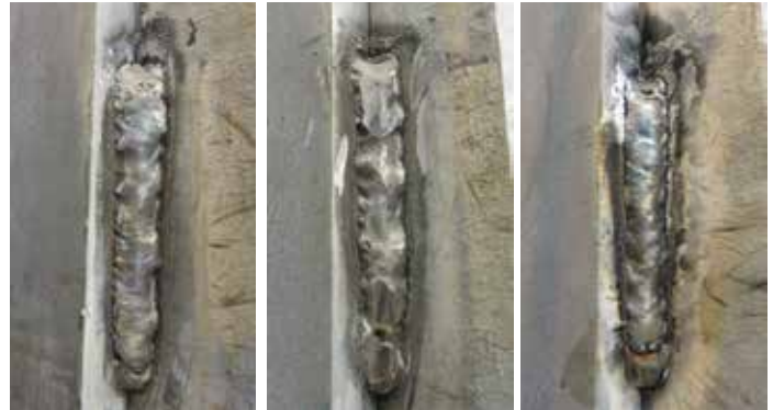
Figure 1. AWS Code D1.1 structural steel welds on galvanized steel – galvanized coating was not removed prior to welding. Numerous welds were rejected due to unacceptable profiles and poor workmanship.
