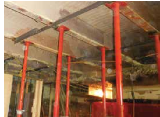
Figure 1. Screw jack set up in preparation for a shore, cut, and reframe scenario.
