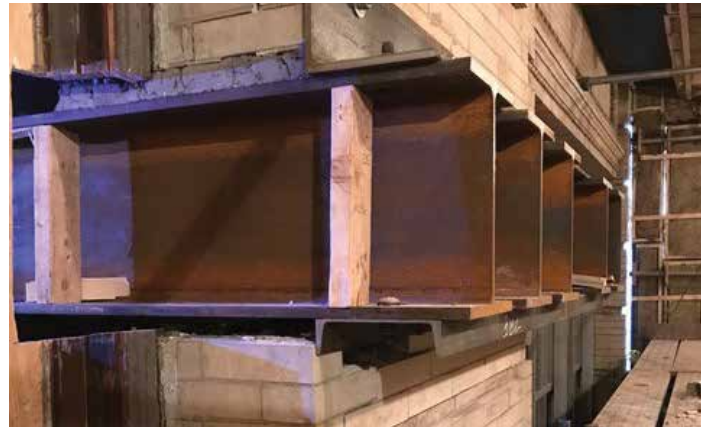
Figure 4. Needle shoring setup. In this scenario, the needle beams are cantilevered from the inside due to site logistics.
