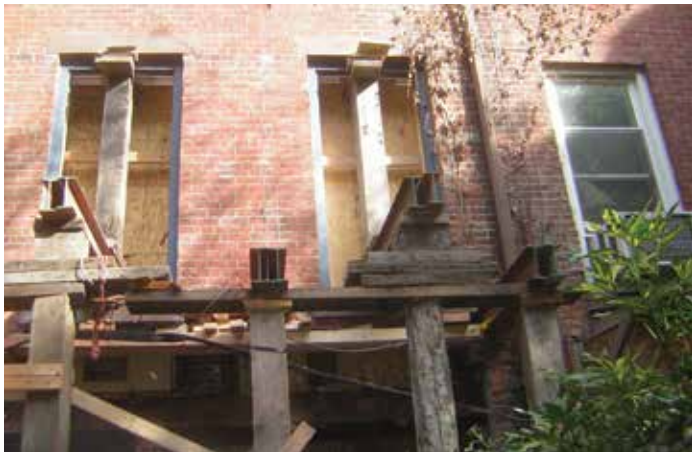
Figure 5. View of rear wall with needle shoring. Note the shoring at the window openings.
