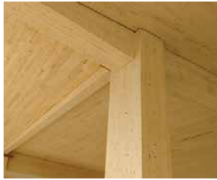
Figure 2. Example fire-protected beam to column connection. Courtesy of Alexander Schreyer, University of Massachusetts, Amherst.
