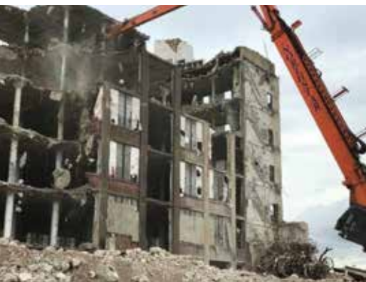
Figure 19. A progressive collapse to the ground floor began on the 4 th floor as a result of overloading the floor framing with an excessively large debris pile.
