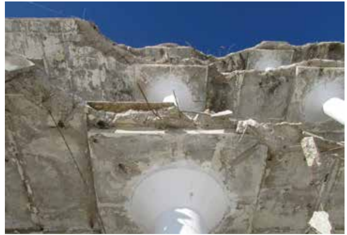
Figure 21. Several top and bottom reinforcing hoops that were intended to remain were destroyed or damaged, resulting in reduced load-carrying capacity of the remaining bays adjacent to the demolition line.
