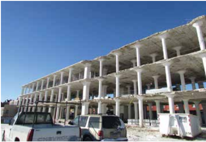
Figure 20. The demolition contractor did not take adequate precautions to ensure a uniform vertical demolition face along most of the eastern line of demolition.
