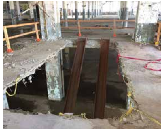
Figure 18. Vehicle access opening cut in the slab during demolition required the installation of shoring posts in the surrounding compromised bays.
