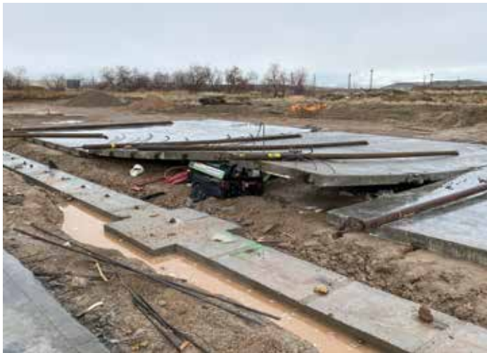
Toppled wall panels thrown approximately 5 to 6 feet.
