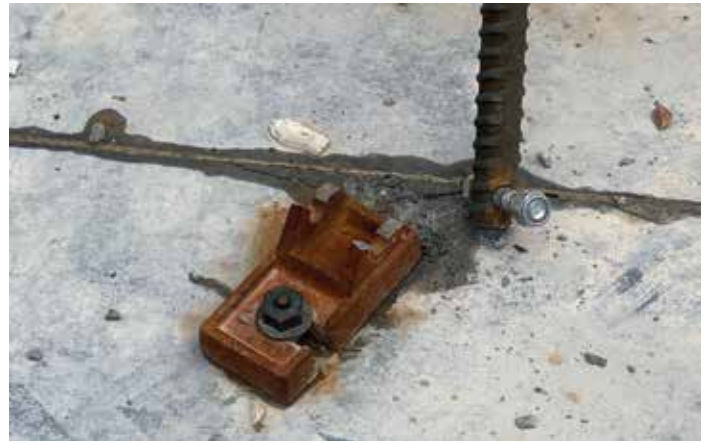
One of several failures of a footplate identified after the earthquake.
